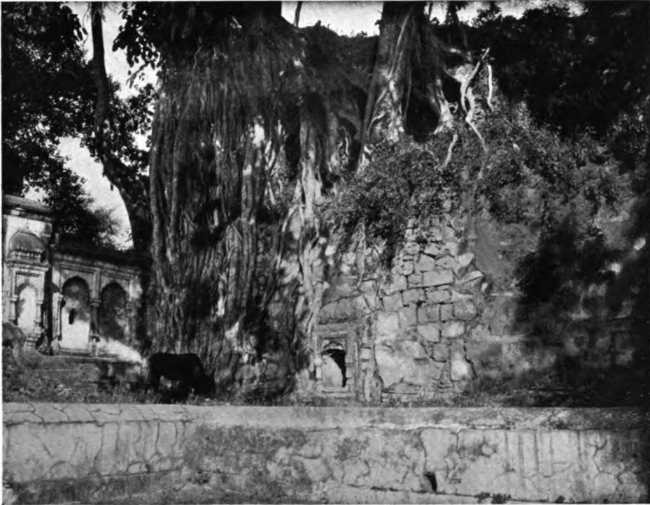
BANYAN ROOTLETS DESTROYING BUILDING, MAHOBA.
